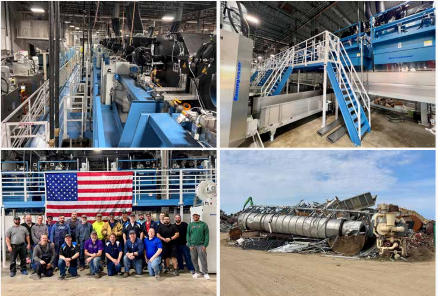
Above: (Clockwise, top/left) overviews of the plant's new dryers. These machines process goods washed in the tunnels; staff were sad to see their old equipment scrapped. But TCS' management, engineering and production teams—plus the Kannegiesser ETECH installers and Carlson Construction crew members shown here—are pleased with the plant's improved performance.
