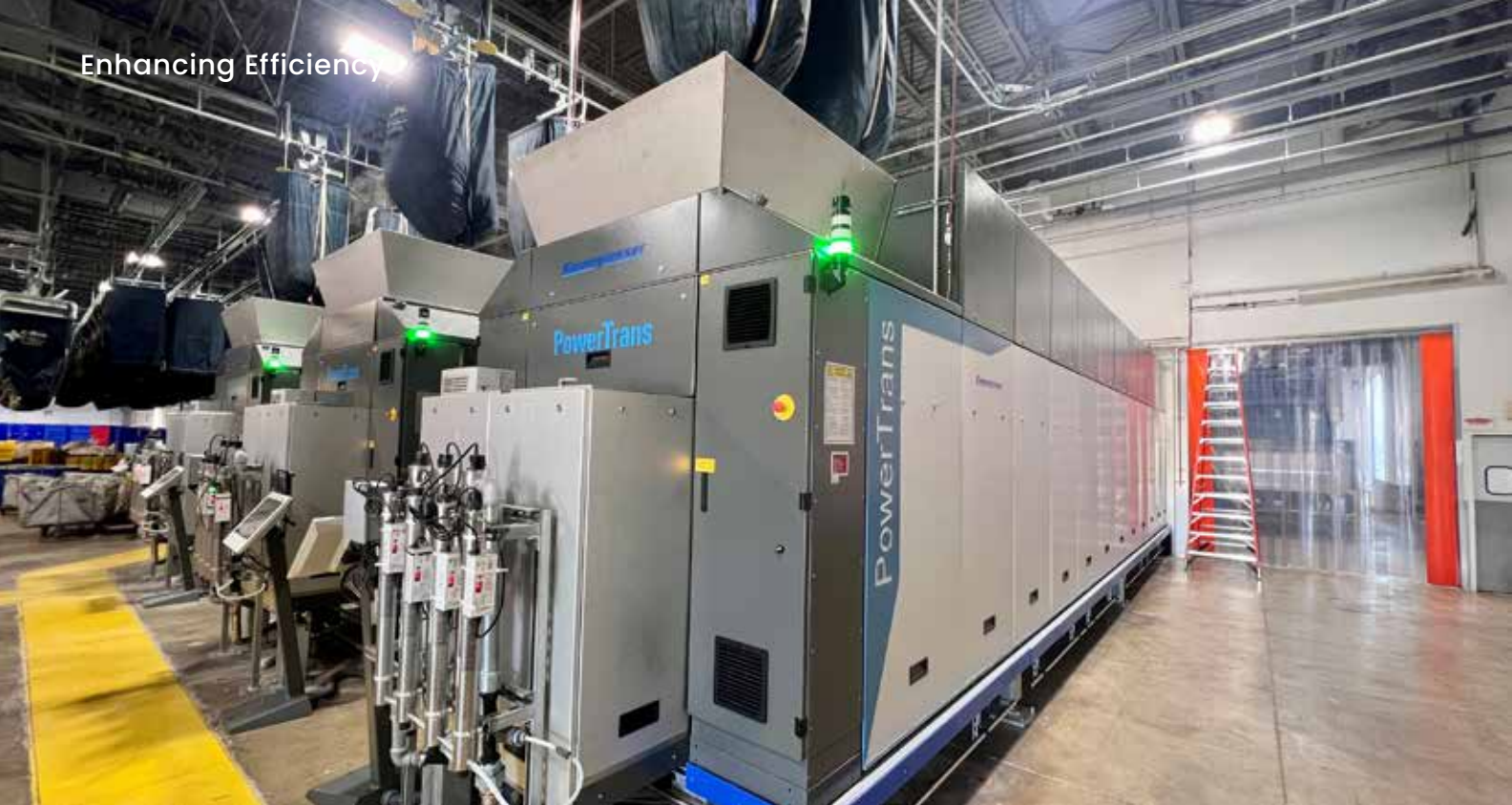
Above: Three new tunnels installed earlier this year at Textile Care Services' healthcare/hospitality laundry in Rochester, MN, have increased efficiency with faster throughput, while providing more effective cleaning of textiles, according to GM Paul Jewison.
